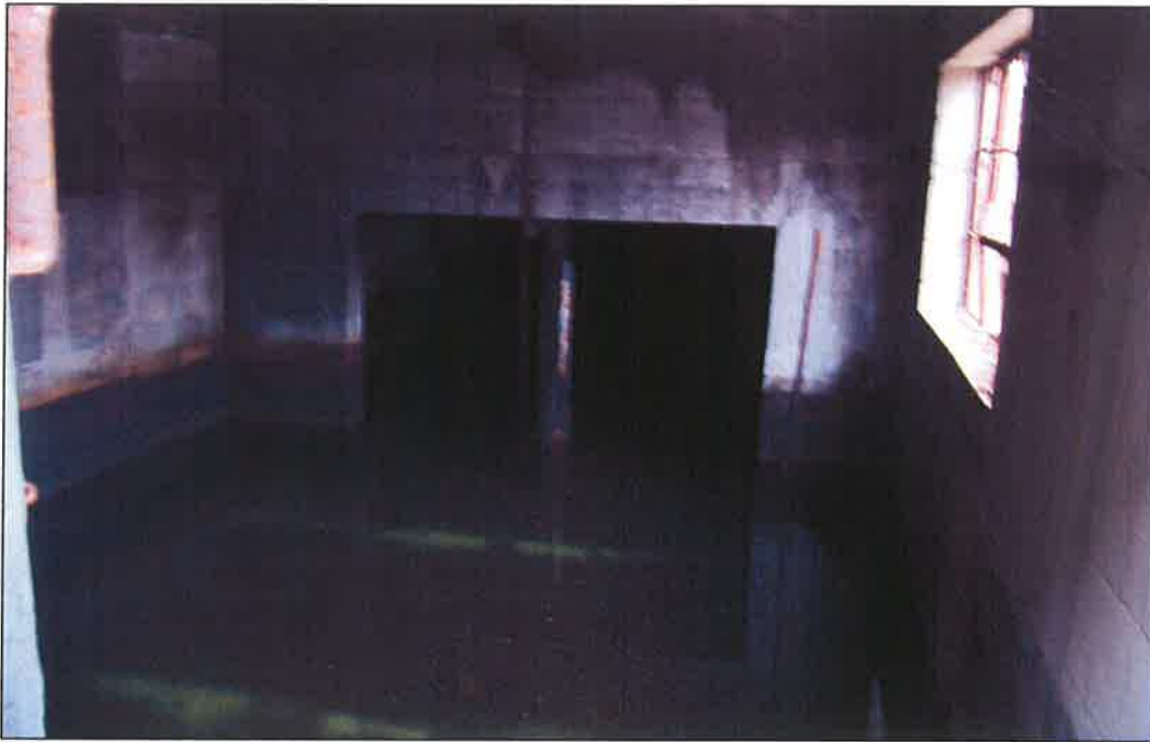
PHOTO NO. 21: Water-filled former boiler room area.
