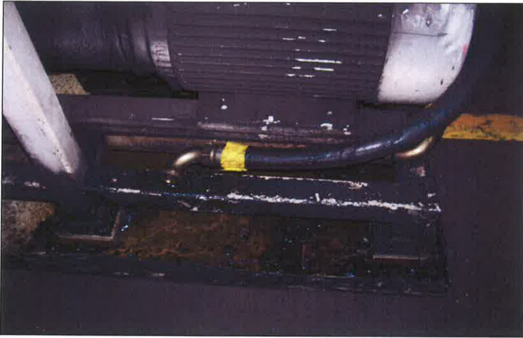
PHOTO NO. 15: Oily machinery stored in building.
