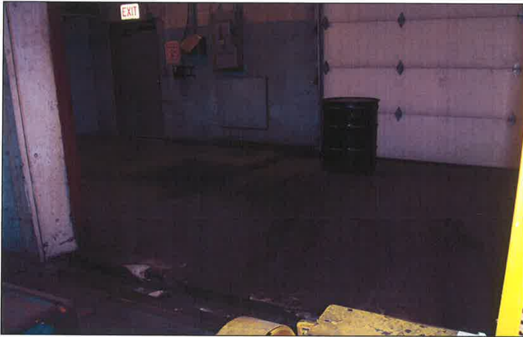
PHOTO NO. 16: Former oil drum storage area, area beneath floor is former boiler room, door to left is alleged TCE dumping area.
